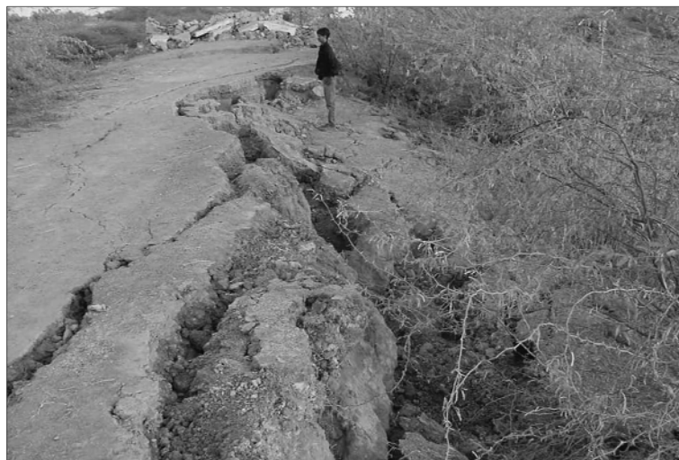
Figure 2. Cracks in earthfill dam following Bhuj earthquake of 26 January 2001
